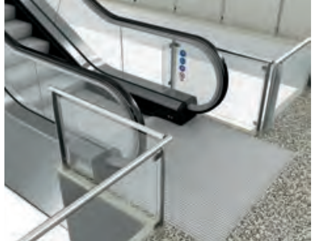
Figure 5.17 Standard arrangement without extended balustrade requires 90° static railings to be installed for safety reasons
